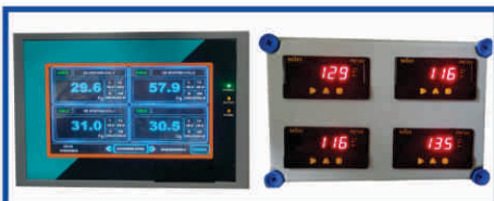
DIGITAL LAW PRESSURE GAS ALARM SYSTEM
